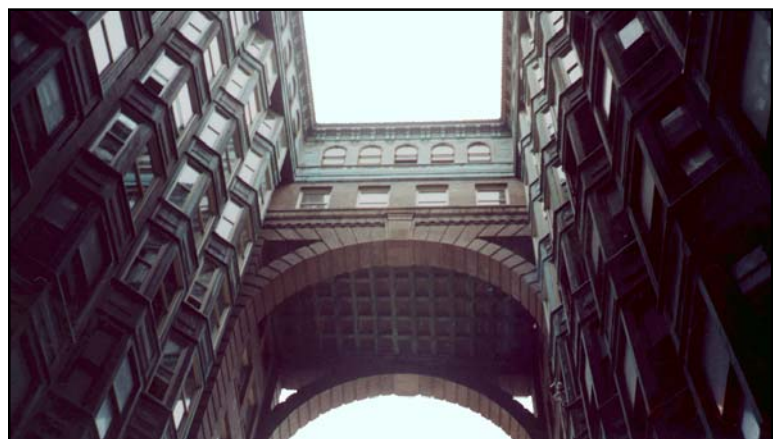
The renovation of the Fulton Building was complicated due to the unusual shape and angles of the facade.
